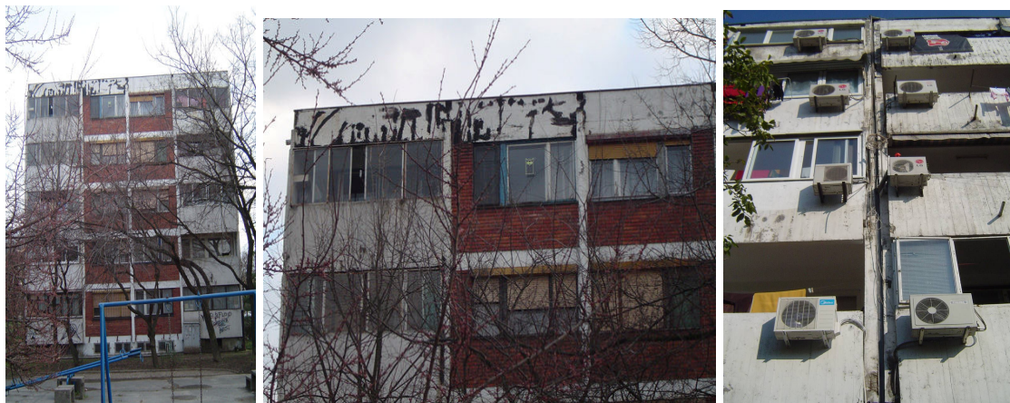
Fig. 9. Façades of the building AP 23-35 with visible damage and outdoor elements of air-conditioning units
